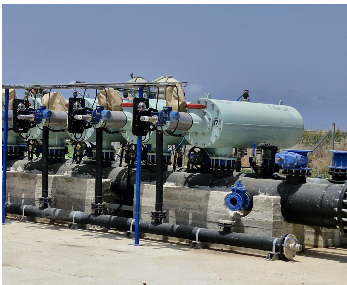
View of installation: 7 TTN 20K Filters.
